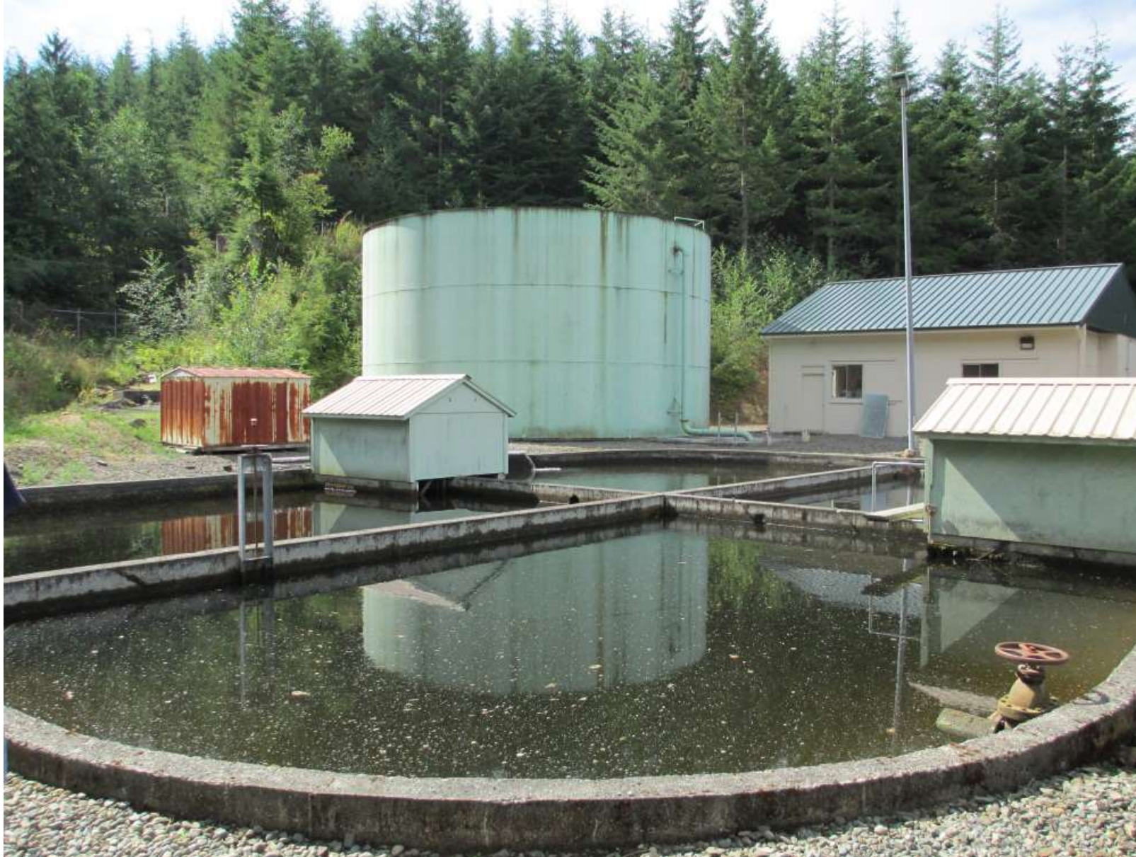
TOWN OF CARONADO WATER TREATMENT FACILITY. SETTLING PONDS ARE IN THE FOREGROUND, TREATMENT PLANT BUILDING IS IN THE BACKGROUND RIGHT, AND CYLINDRICAL FINISHED WATER STORAGE TANK IS IN BACKGROUND CENTER.
