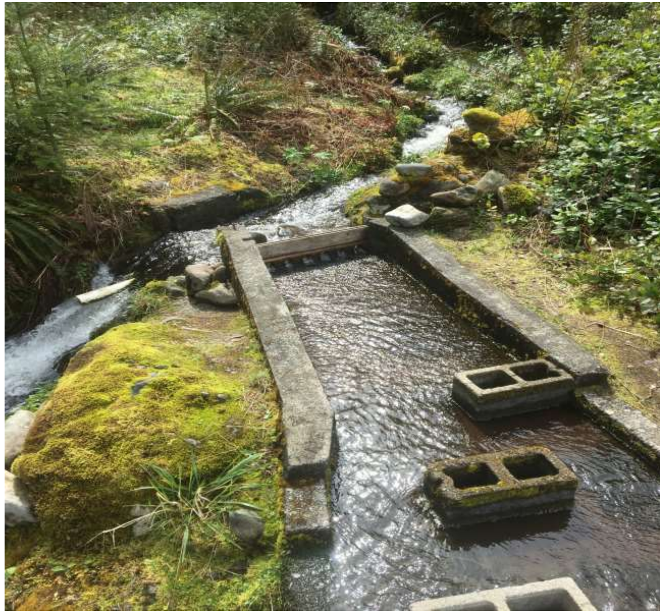
Little Camp Creek intake collection box looking upstream to water source
