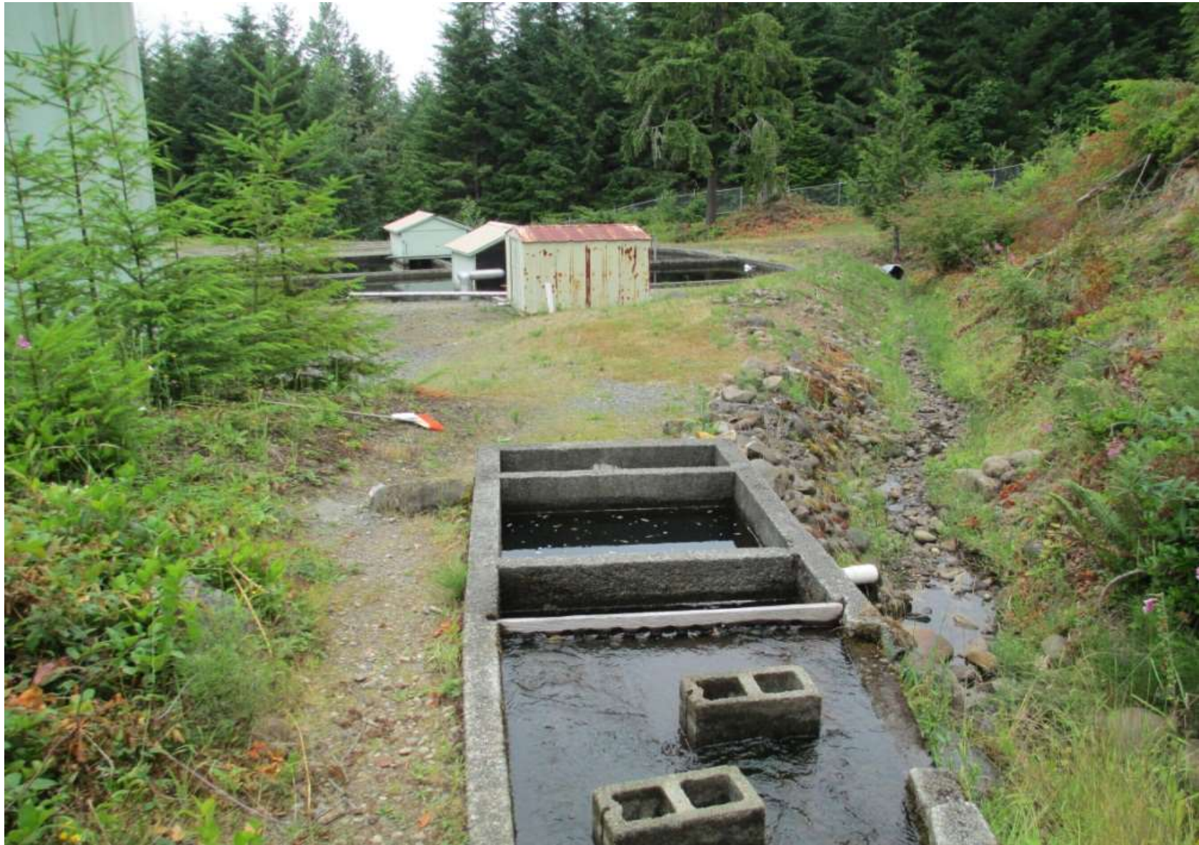
Little Camp Creek intake collection box looking downstream to water treatment facility and the pipe (at raw water reservoir) for the North Lines (used during summer months)
