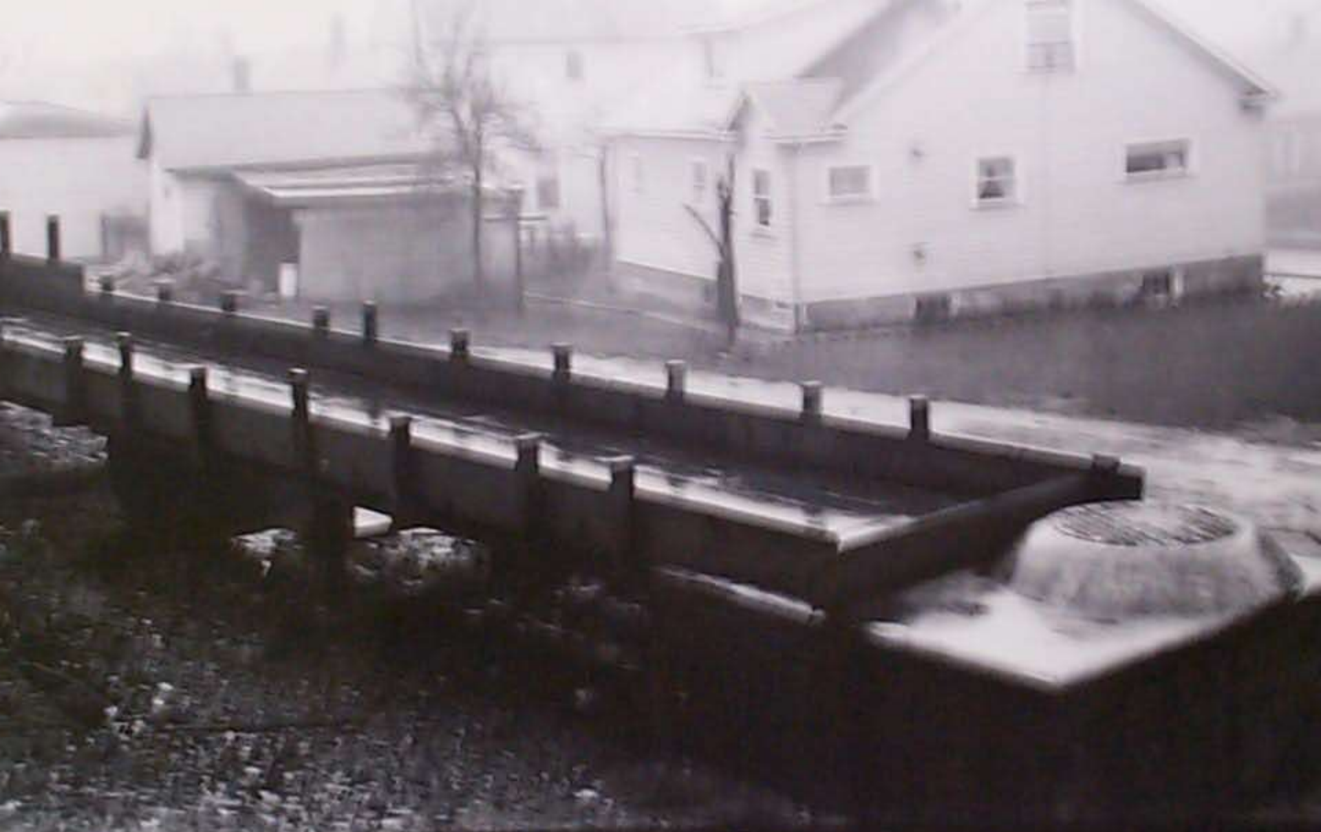
26-Hallat - Well 5A - Discharge Flume
