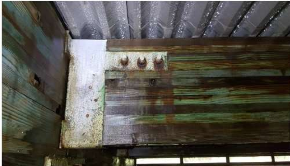
Typical Corroded Purlin Hanger
