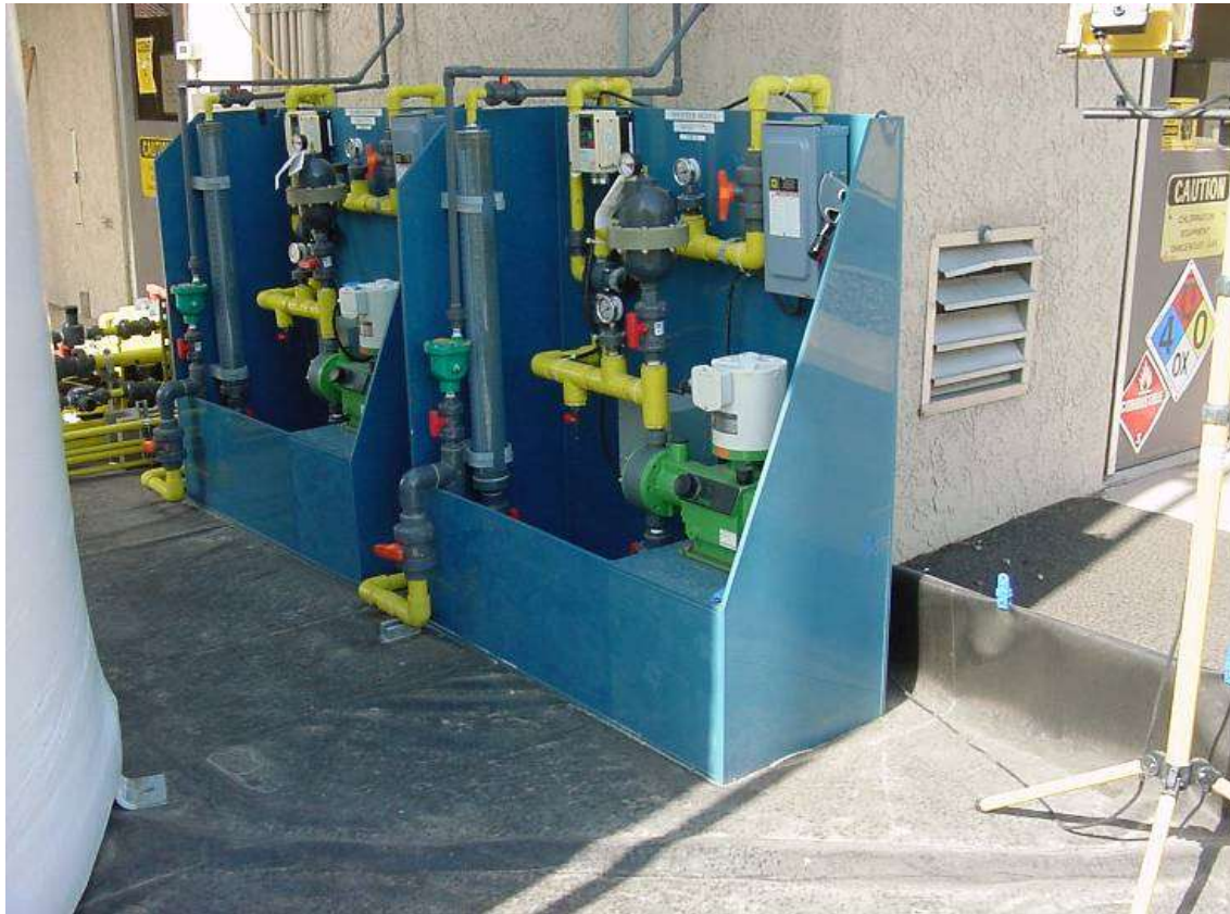
Typical Sodium Hypochlorite Dosing Station
