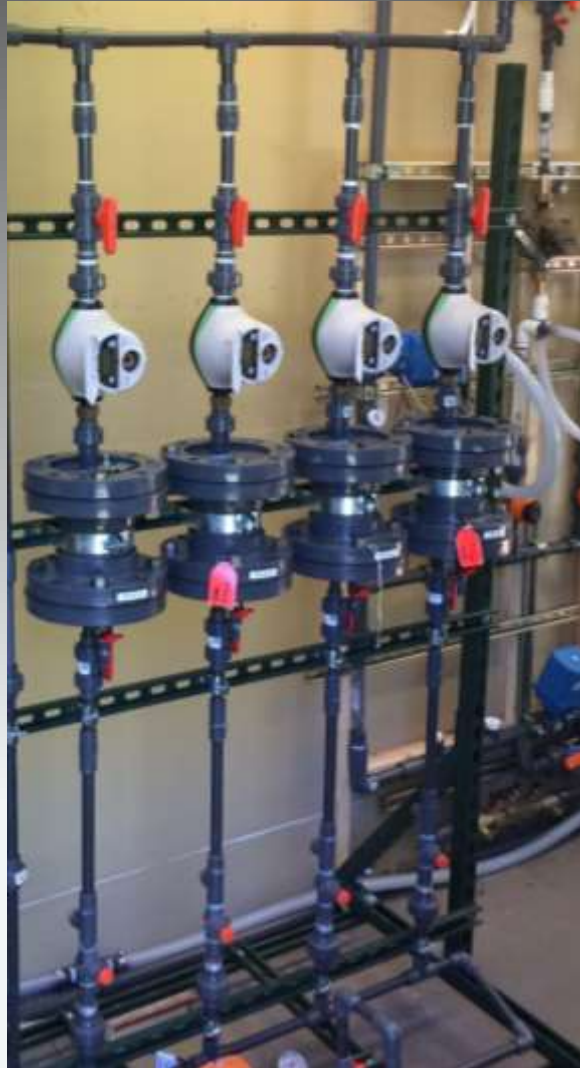
4-Chamber PRS Station
