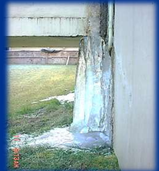
Ice formed outside Water Holding Structures (from leaks)
