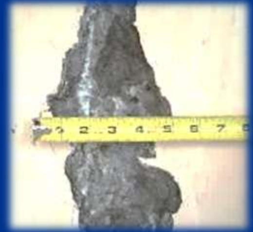
Spalling of Water Holding Structures
