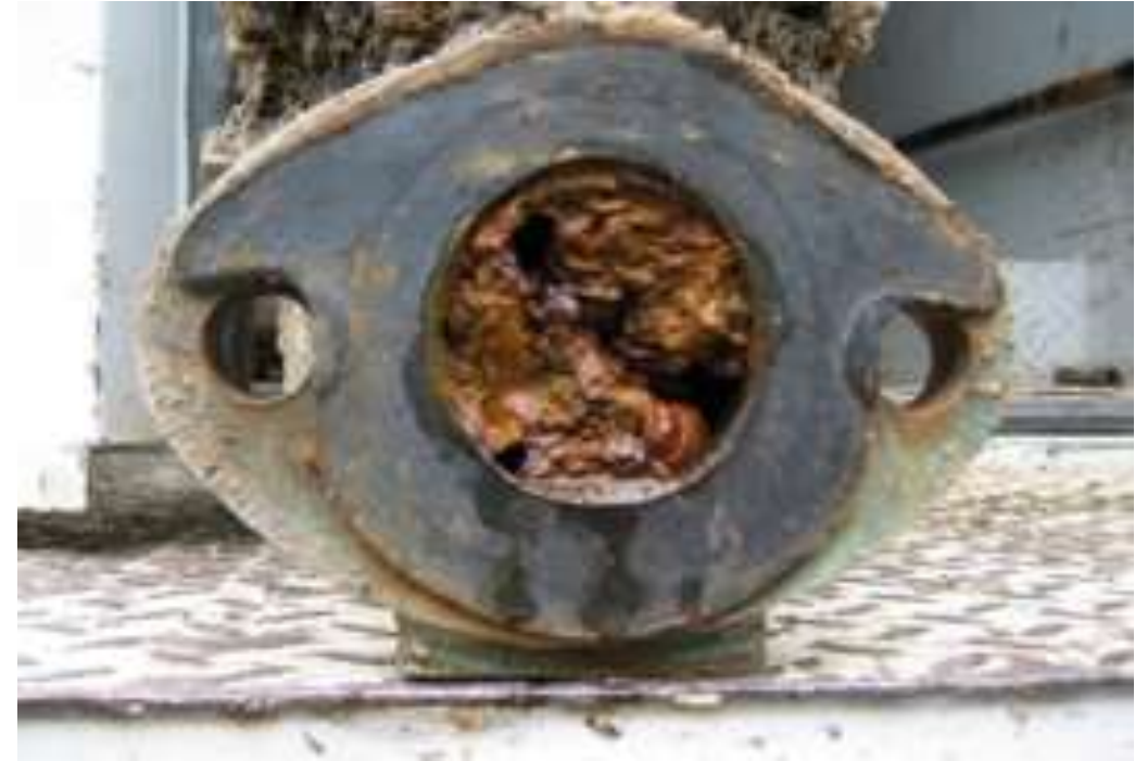
2-inch service line
