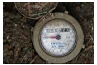
Customer meter under registration
