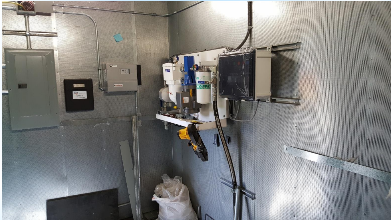
Fuel Conditioning System
