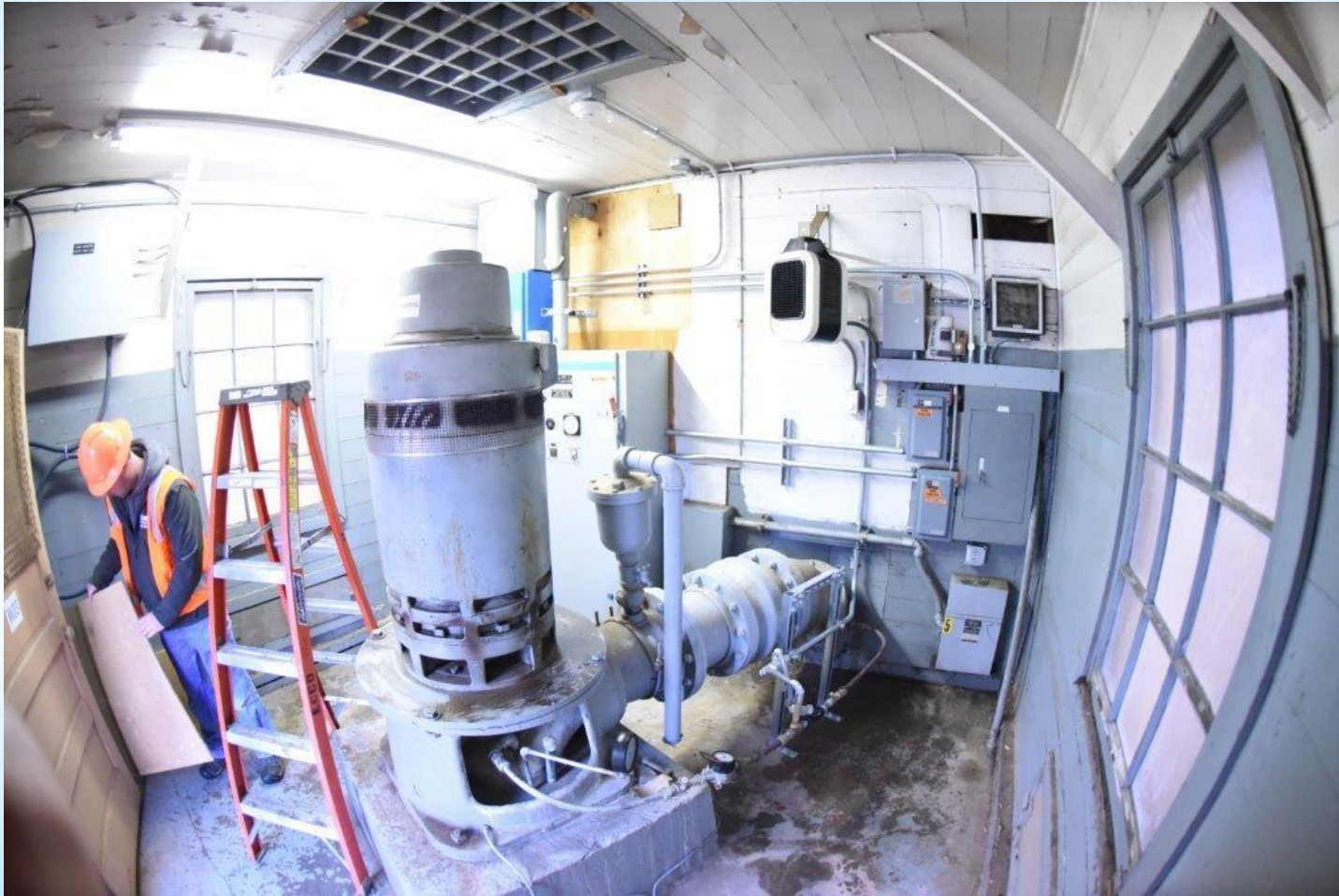
Inside Well House 3
