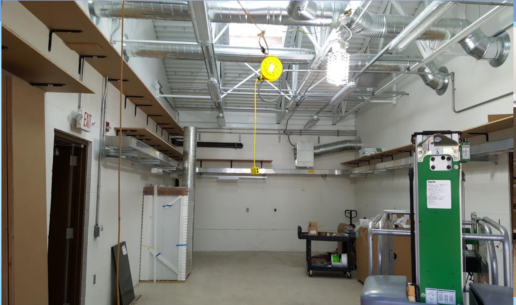
Redundant Server Room, Control Room, SCADA Shop
