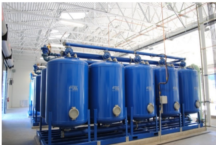
Southlake Water Treatment Plant
