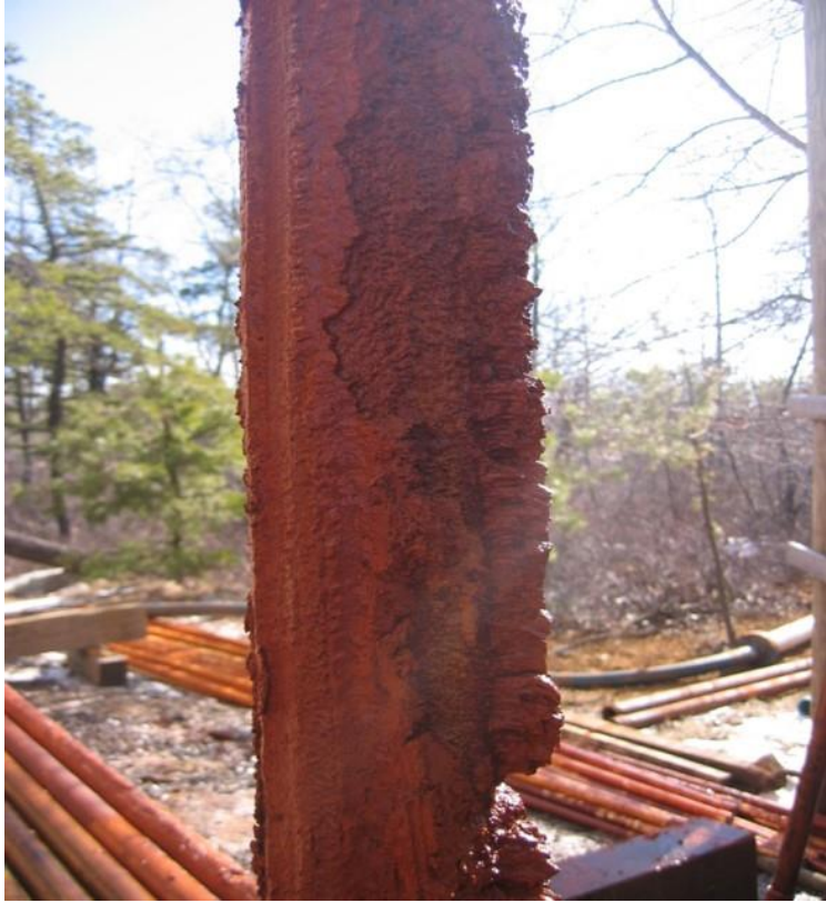
Plugging on exterior of well screen
