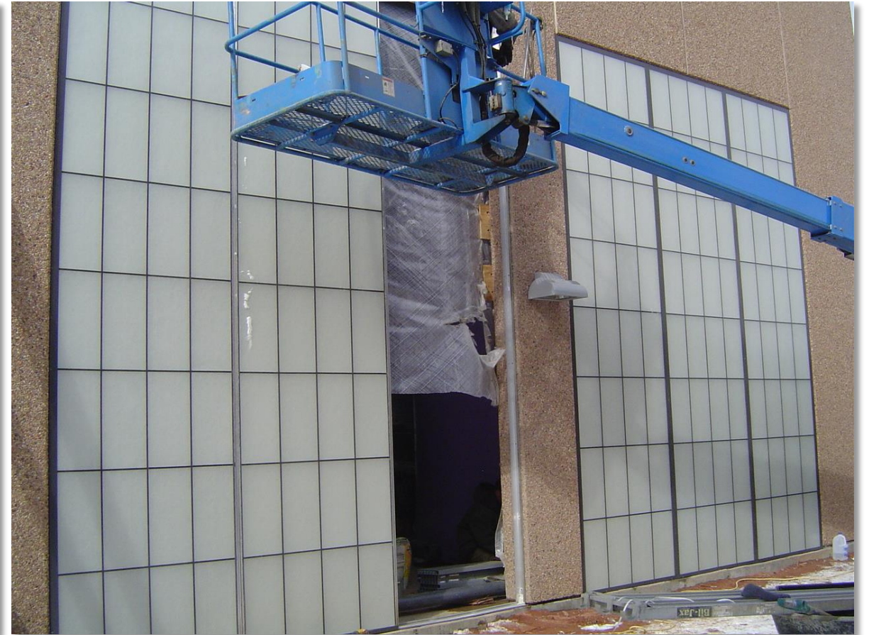
Removable wall panels and rollup doors
