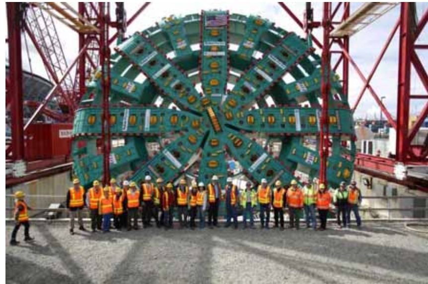
Cutter head for Bertha – tunnel boring machine for Seattle’s State Route 99 Tunnel. Repairing damage to the TMB delayed the project three years
