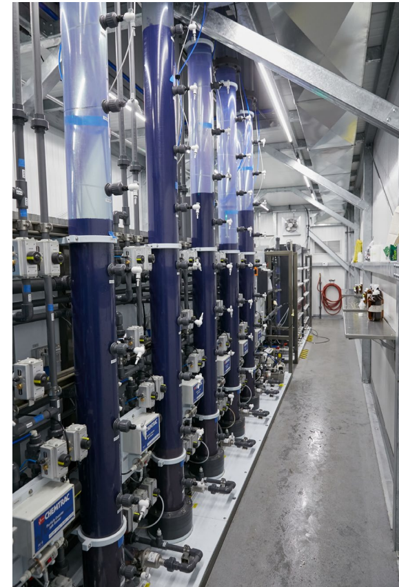
Bull Run Pilot Plant Filter Columns
