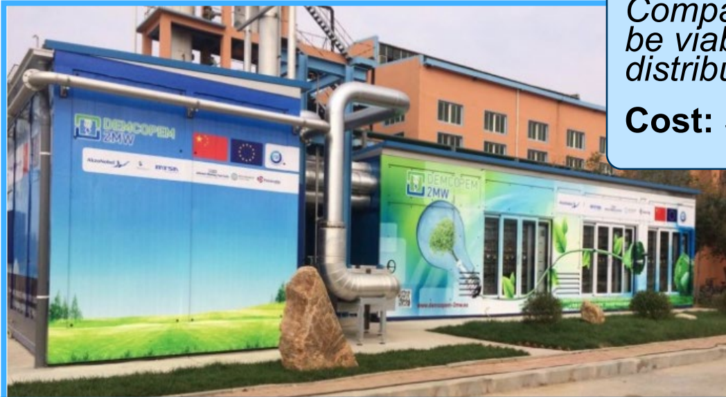
Demonstration 2MW Hydrogen Fuel Cell System
