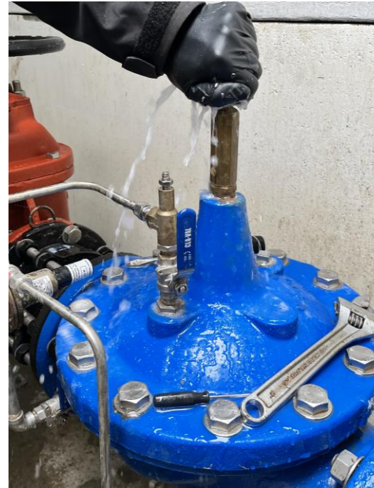
Maintenance, troubleshooting, startups
