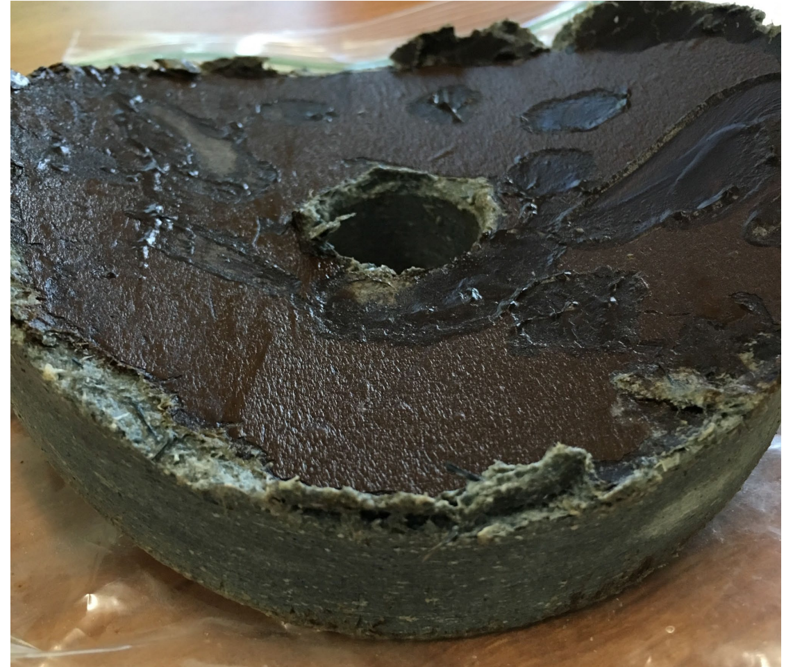
Asbestos Cement Pipe Utah system
