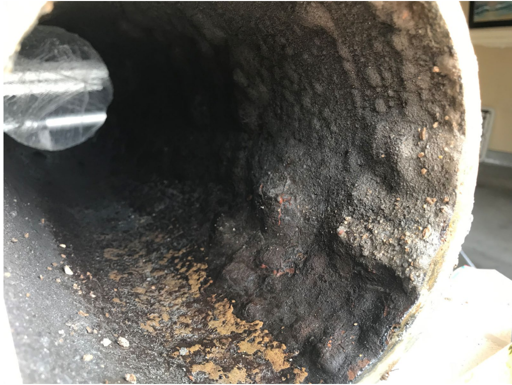
Unlined Cast Iron Pipe Idaho system
