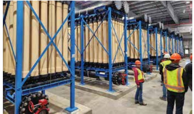
New membrane skids provide tertiary treatment, referred to as Next Level of Treatment, to reduce nutrients and pollutants of water released to the river.
