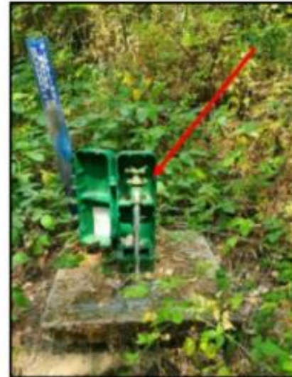
Valve at 24-inch
