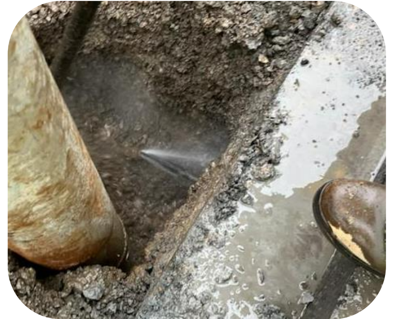
Identify and repair the leak(s)
