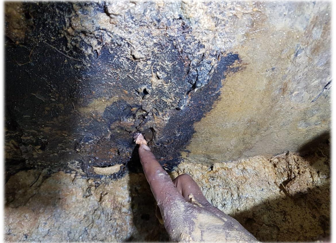
Leak Plugged with Wood Splint Smaller than Finger
