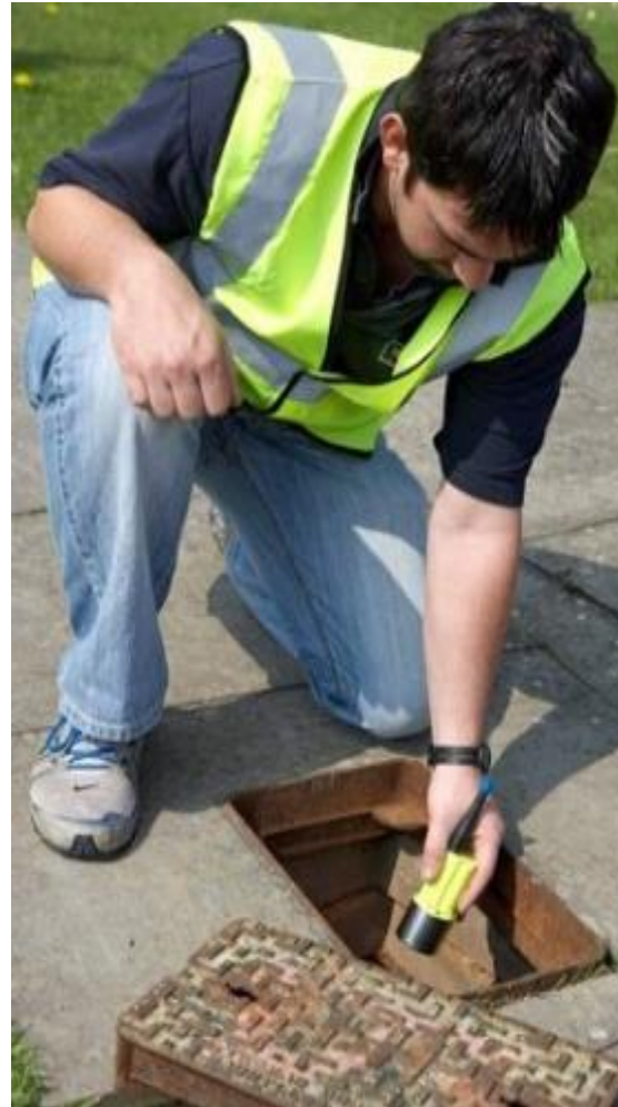
Lift-&-Shift Noise Loggers
